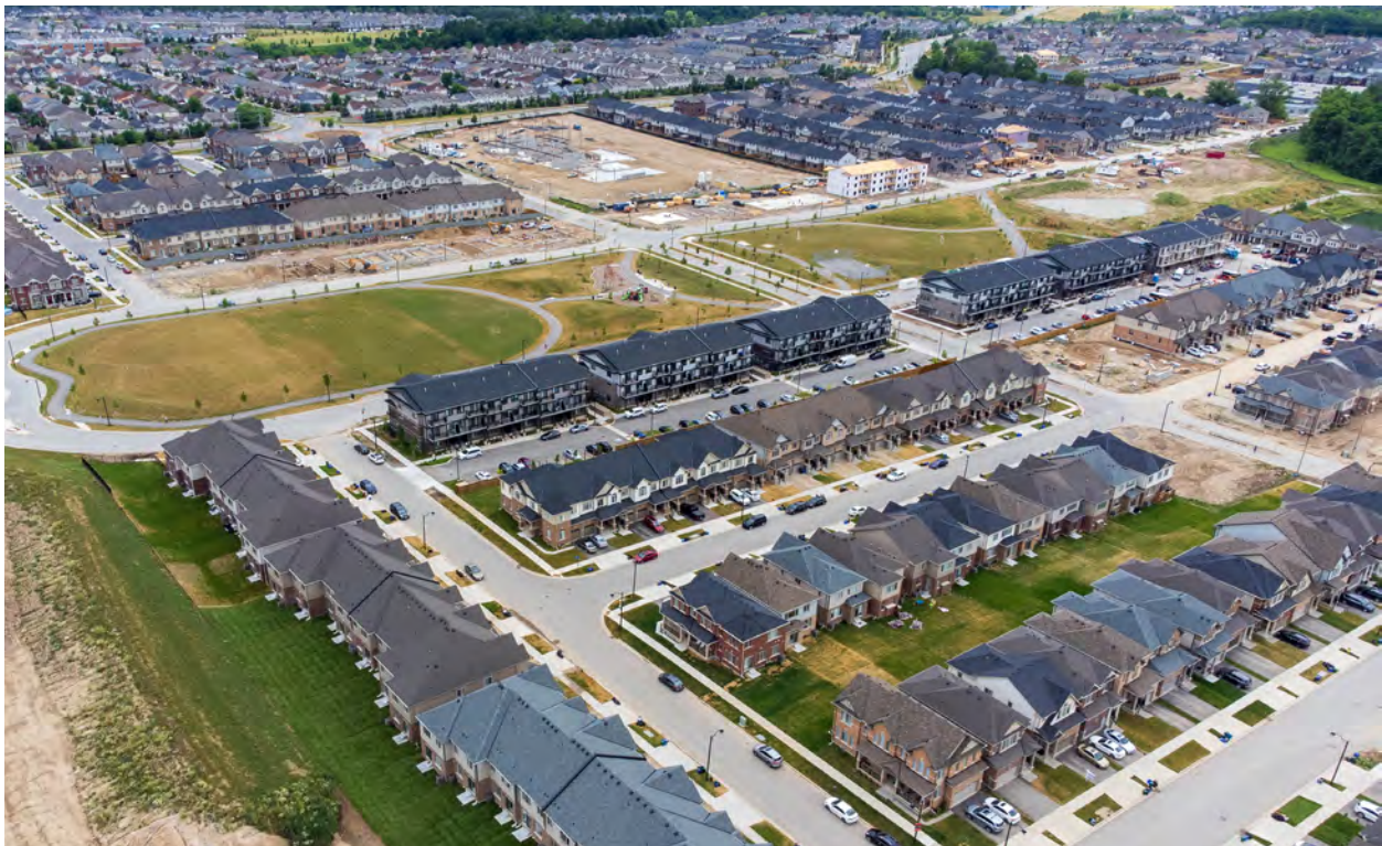
Figure 8: Construction at Schlegel's Wallaceton community. A full range of housing including detached forms and street and stacked townhomes are under construction along with a new elementary school.
