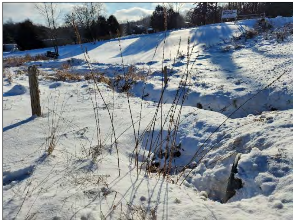
Photo 12. Twinned outflow culverts adjacent to the Subject Property, on the opposite side of County Road 25 (December 21, 2022).
