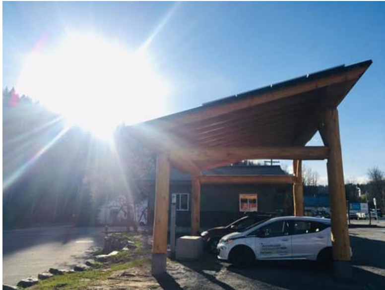
Solar PV array installed atop car park cover at Kimberly Platzl
