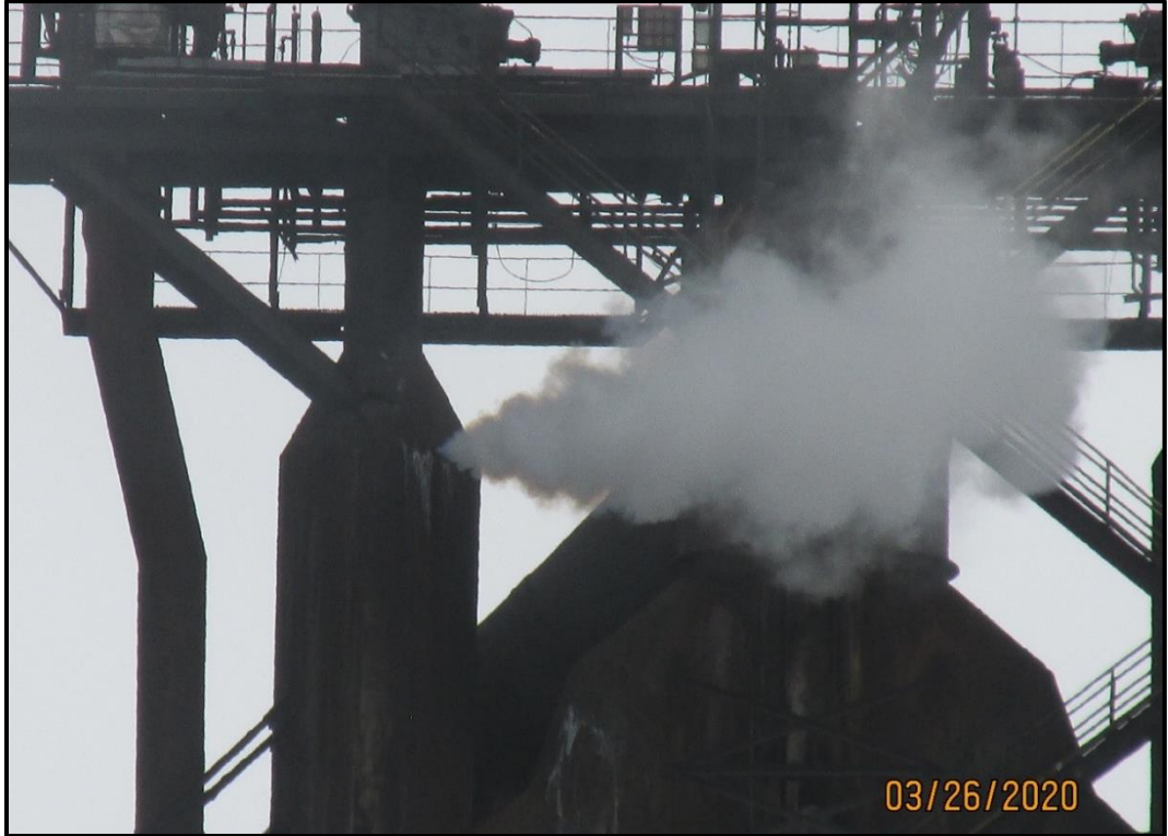
Photo 3: Typical appearance of dirty emissions from the leak @ 1:48 pm from Bonney St.
