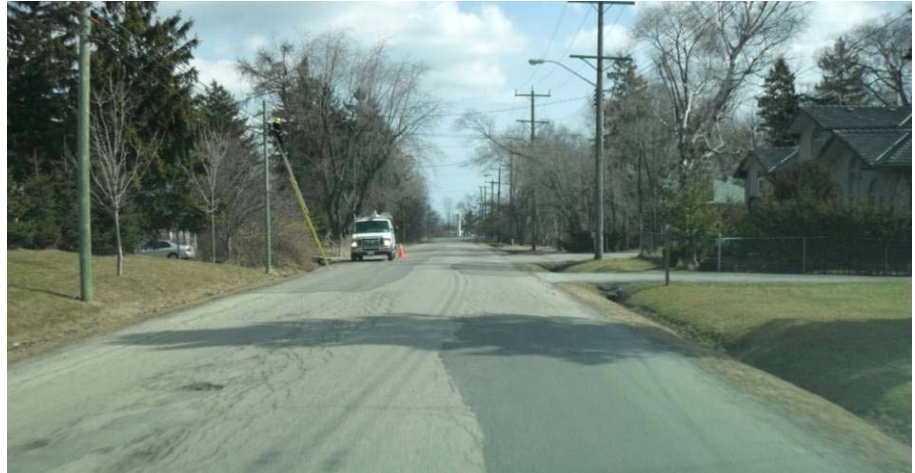
Figure 3. Alligator Cracking and Patching on Beechgrove Drive
