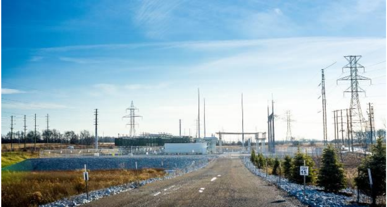
Figure 3: A Typical 230 kV Transformer Station
