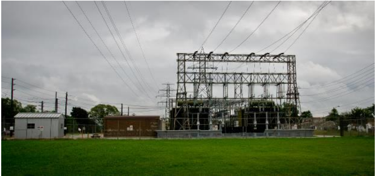
Figure 4: A Typical 115 kV Transformer Station
