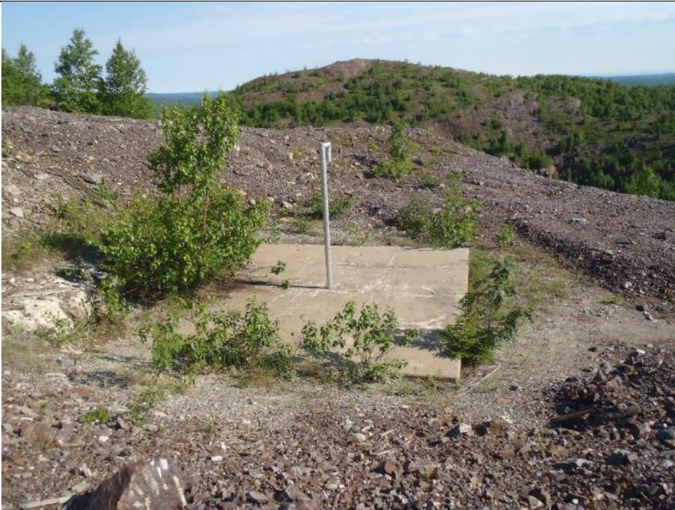
Photo 3: H221 Fresh Air Raise within the fenced area. Facing northwest.
