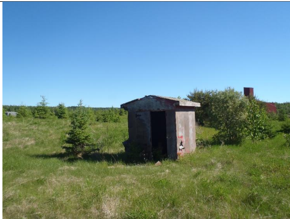
Photo 44: Fire Hydrant Hut condition has deteriorated since the last inspection. Facing north.
