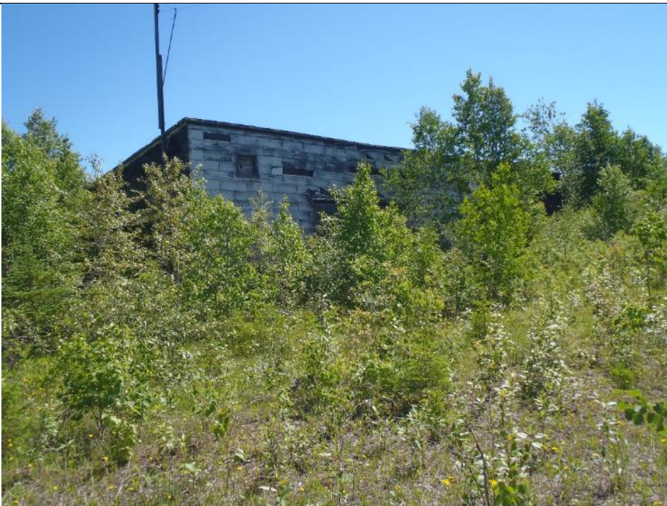
Photo 36: Cold Storage building showing siding falling off. Facing east.
