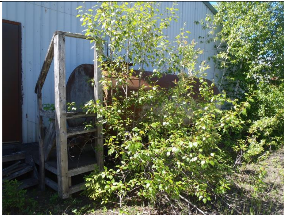
Photo 80: Diesel tank on north side of the Warehouse building. Facing southwest.
