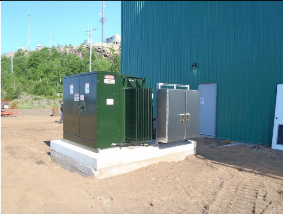
Photo 75: New transformer adjacent to Water Treatment Plant. Facing northwest.
