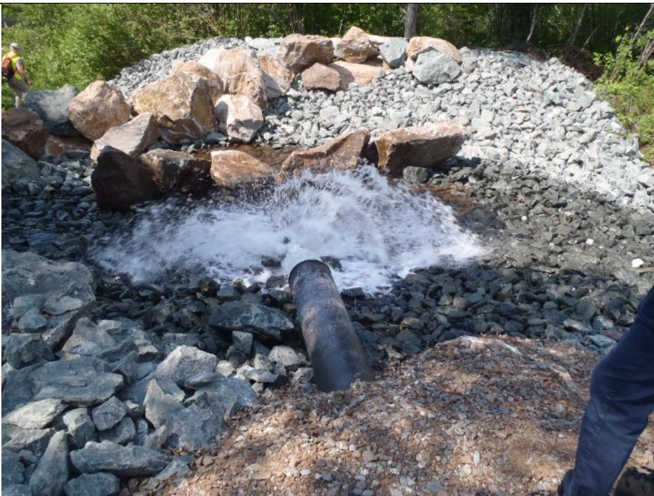
Photo 26: Final discharge point for water treatment plant on the Magpie River. Facing southwest.
