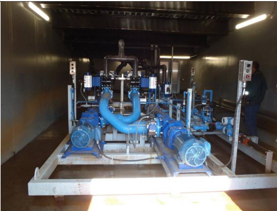
Photo 70: Water Treatment Plant Clarifier interior showing recycling pumps and waste water pipe to Boyer Lake on far right. Facing northwest.
