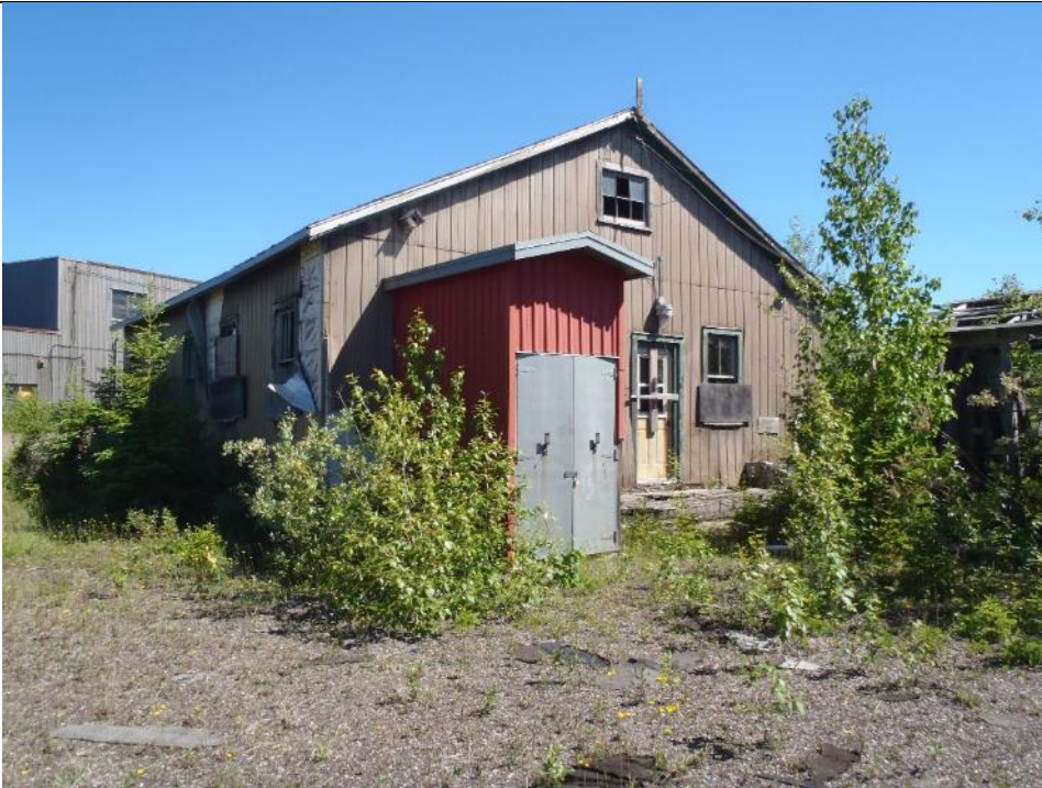
Photo 35 : Carpenter Shop condition has deteriorated since last inspection. Facing north.
