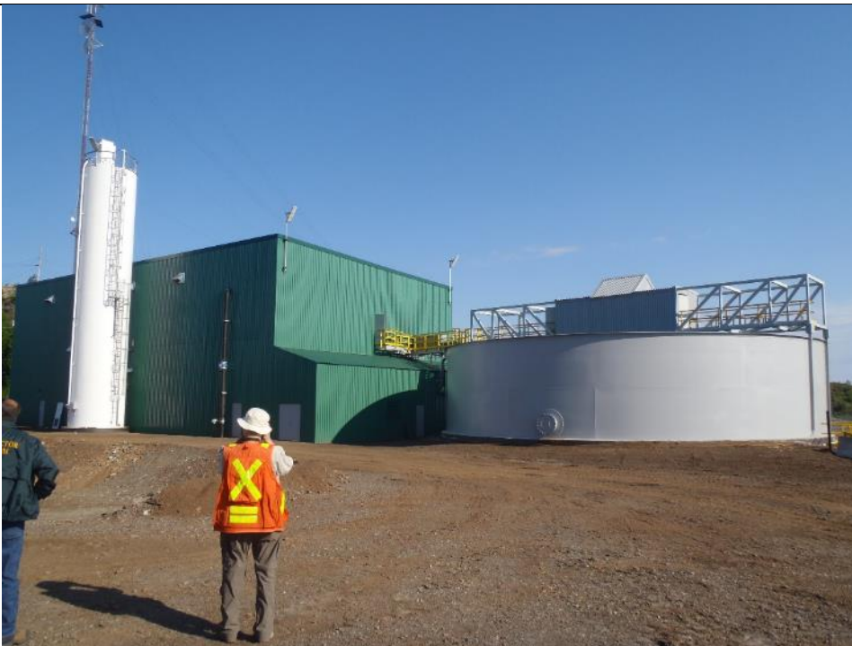
Photo 66: Water Treatment Plant, Lime Silo, and Clarifier. Facing west.
