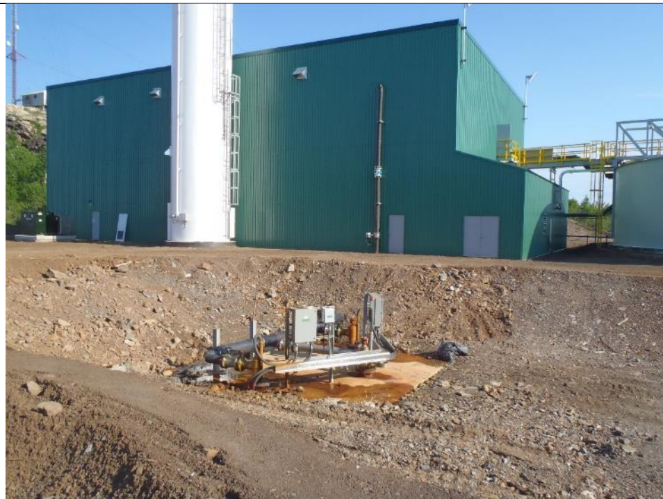
Photo 78: Three new pumps to service the Water Treatment Plant. Facing northwest.
