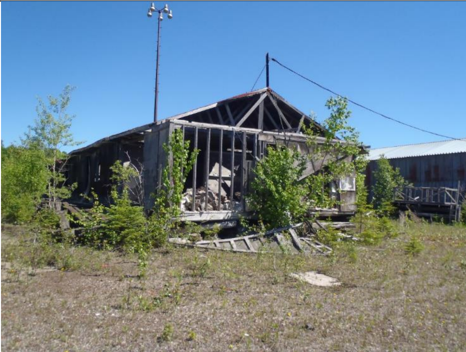
Photo 61: Screen Shed, very unstable. Facing northeast.
