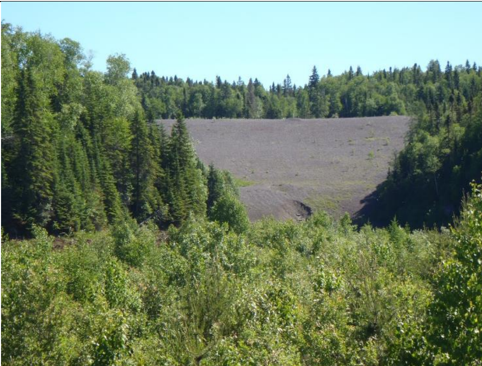
Photo 14: Slump of material on toe of Upper Dam. Facing northeast.
