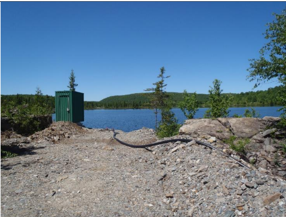
Photo 74: Moran Lake Pump house and waterline to Water Treatment Plant. Facing northwest.
