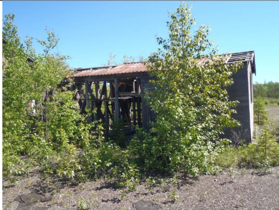
Photo 63 : Tool Storage Shed, very unstable. Facing northeast.
