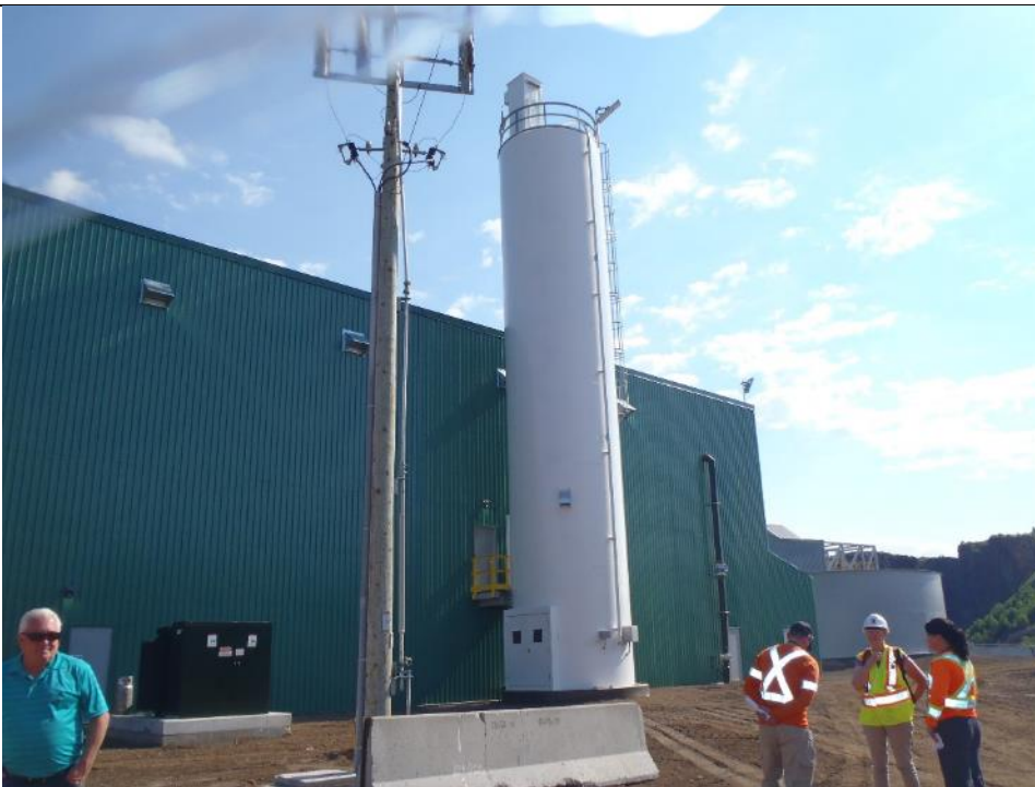
Photo 82: Lime silo adjacent to Water Treatment Plant. Facing northeast.
