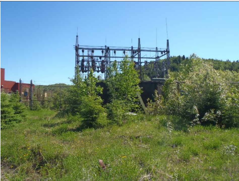
Photo 76: No. 5 Substation on Sinter Plant site. Facing north.
