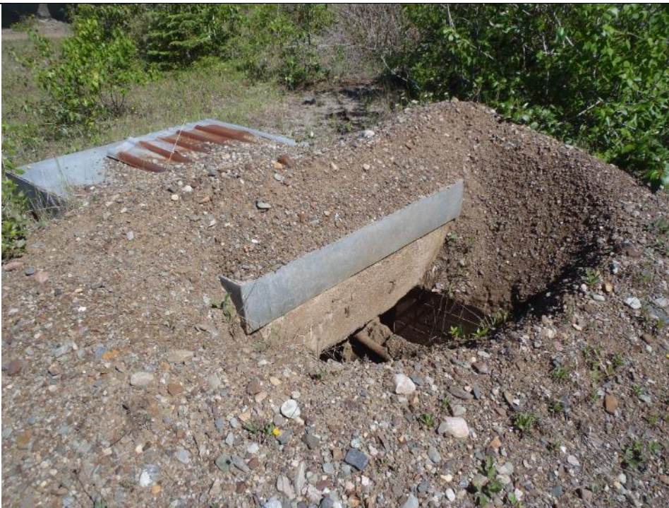
Photo 8: End of Josephine Tunnel showing subsidence of fill material. Facing northwest.
