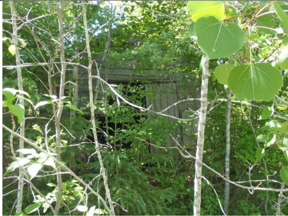
Photo 33 : Brick Storage shed is very unstable. Facing west.
