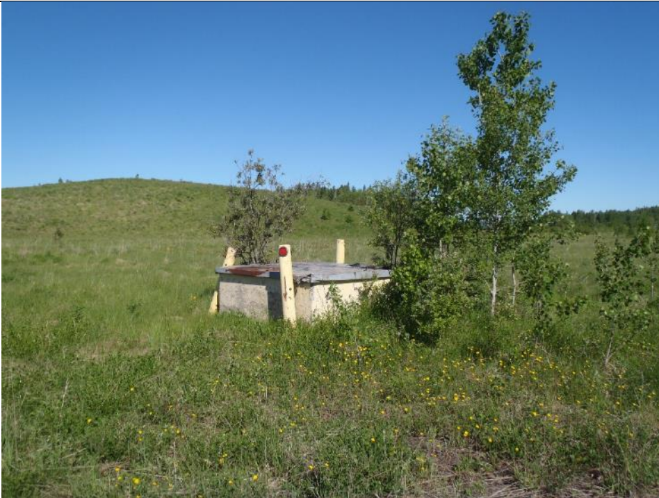
Photo 65: Utility Box on Sinter Plant site. Facing north.
