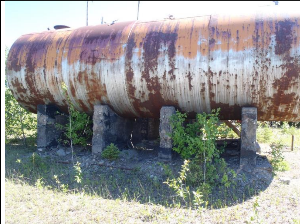
Photo 79: Oil tanks at the Compressor Boiler House showing deterioration of the tanks and concrete base. Facing northeast.
