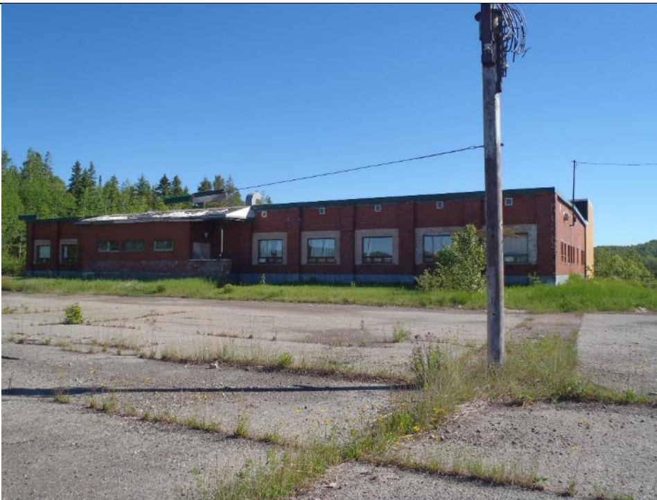
Photo 32: Administration building has deteriorated since last inspection. Facing north.
