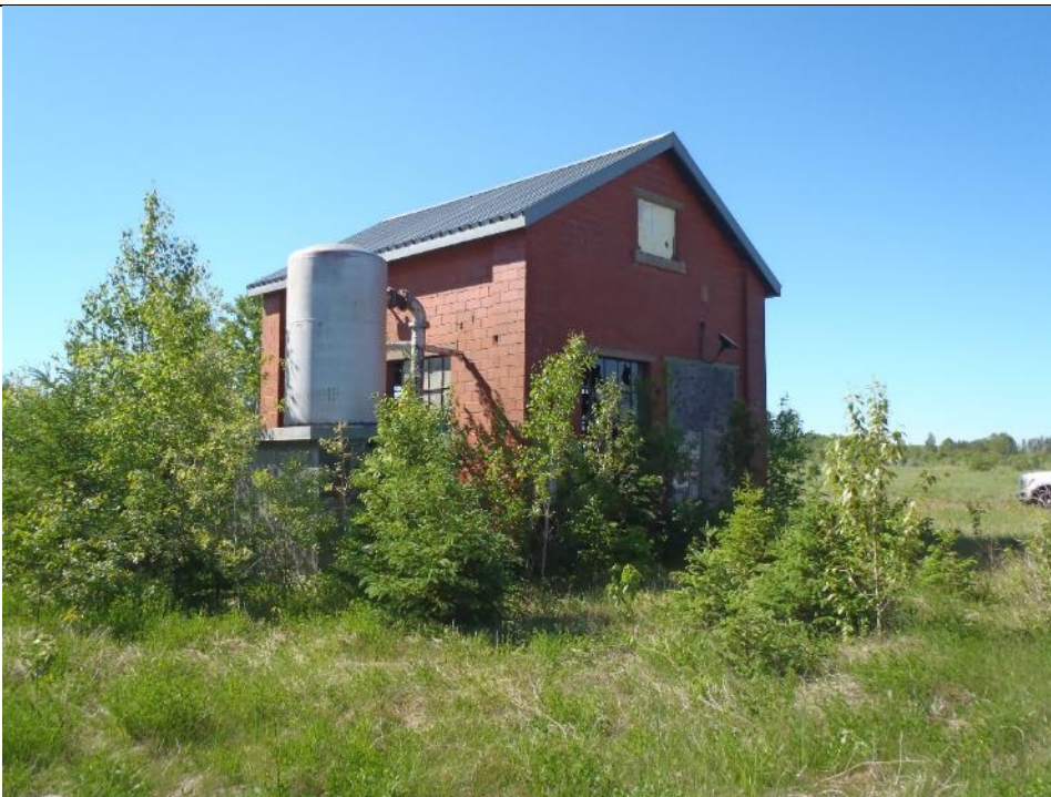
Photo 38: Compressor House showing broken and boarded windows, fuel tank. Facing south.
