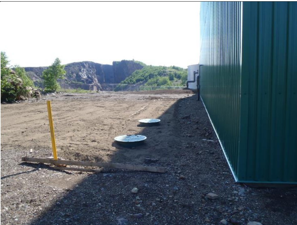
Photo 84: Septic tanks located on the northwest side of the Water Treatment Plant. Facing northeast.
