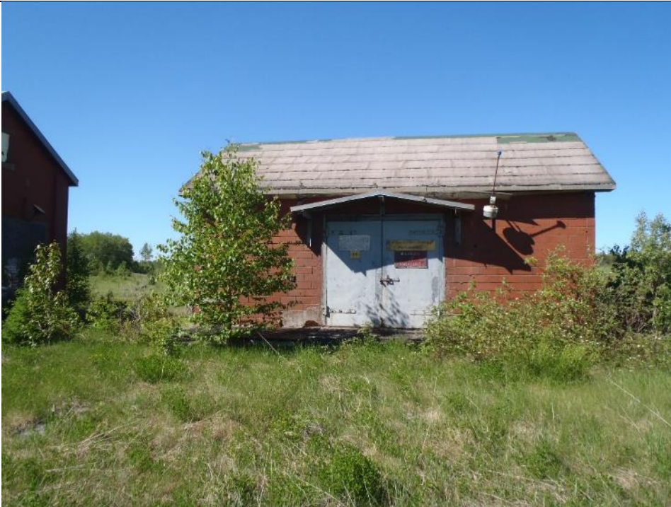
Photo 55: Oil Shed. The windows are broken and some shingles are missing. Facing south.
