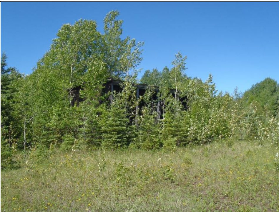
Photo 62: Tire Storage Shed. Surrounding vegetation denser than at last inspection. Facing west.
