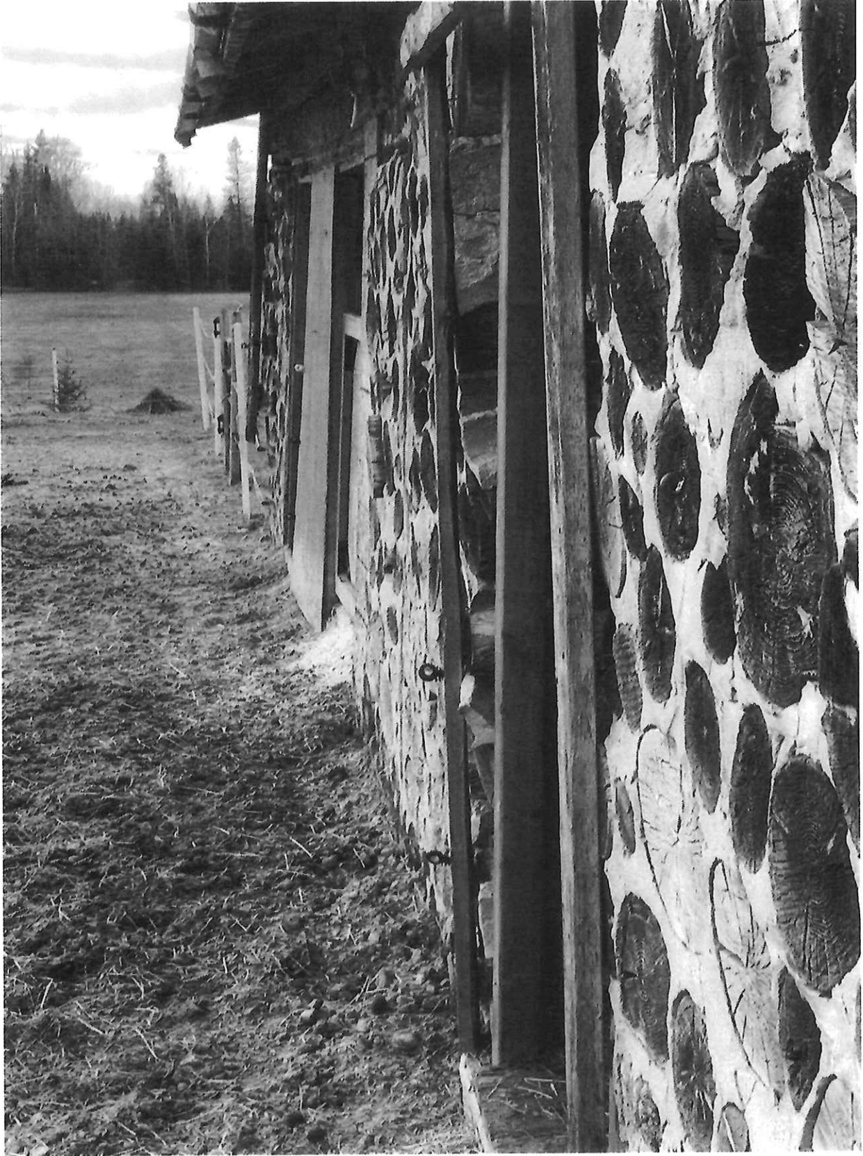
dilapidated barn / shed / stable Entire south wall caving inward.
