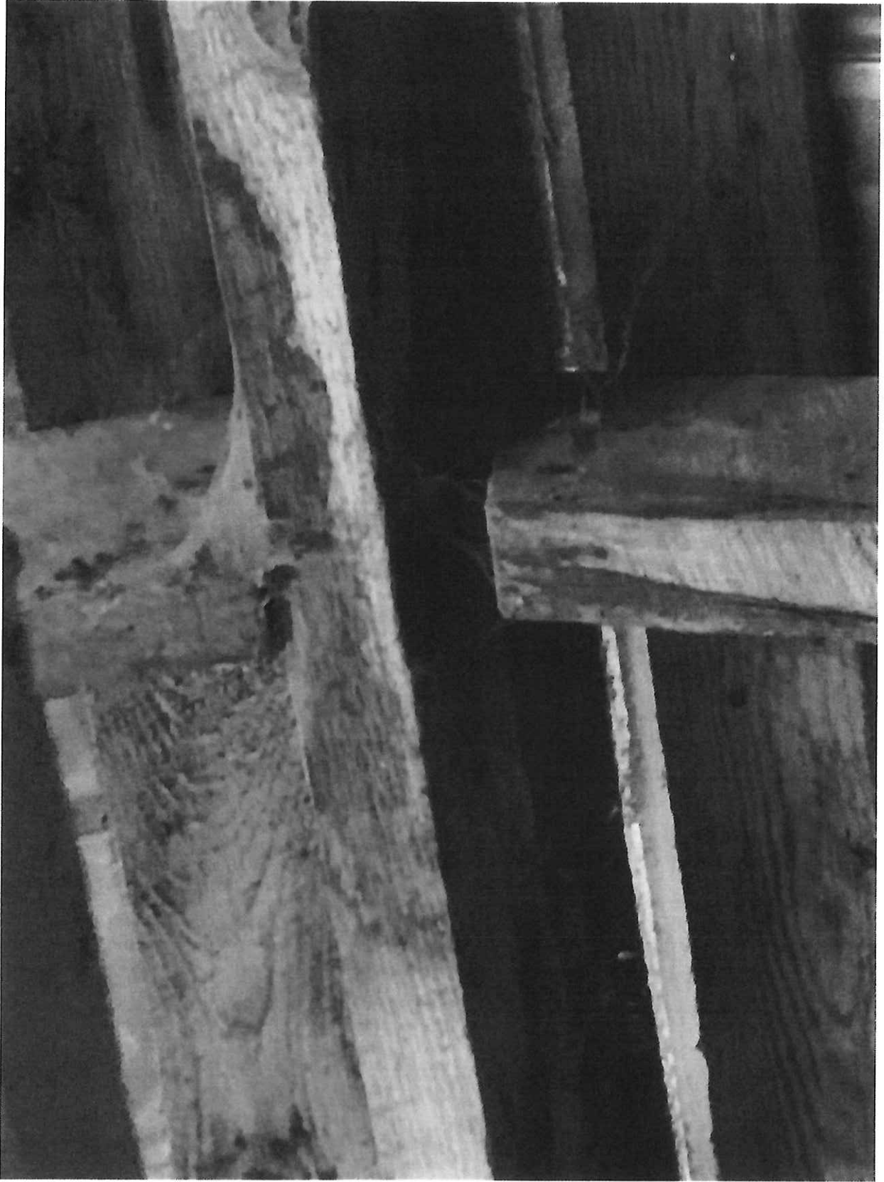
dilapidated barn / shed / stable Roof rafters are pulling apart.
