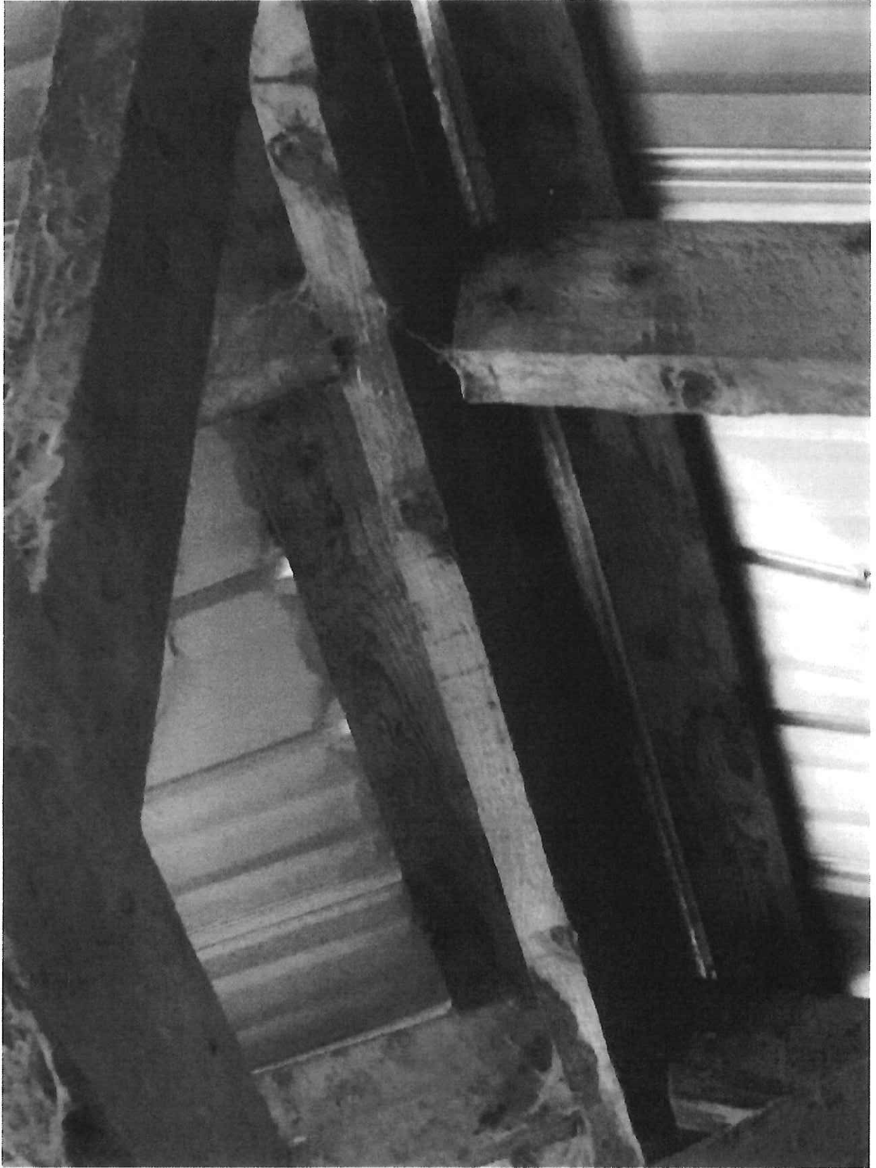
dilapidated barn/shed/stable Roof rafters are pulling apart
