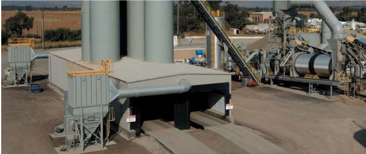
Figure 3 Example of a vapour recovery system which includes enclosure of the loadout point.
