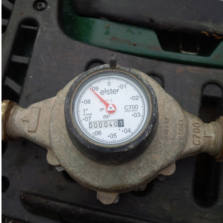
Photograph No. 1 In-line Flow Meter used for pumping tests at MW7 & MW8
