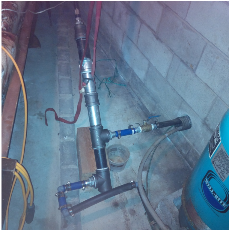
Photograph No. 4 – PW2 In-Line pipe in which a data logger was installed
